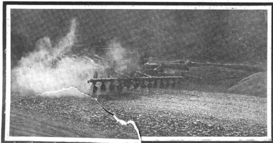
Splendid view of machine used in Massachusetts for spraying hot oil under pressure upon roads
